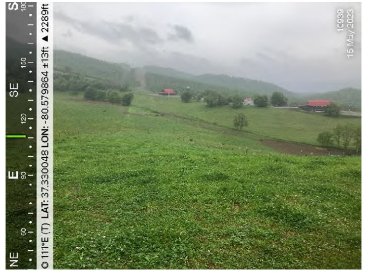
Figure 4: STA 10939+00 – Permanent vegetative cover established. Ground cover is uniform, mature enough to survive and will inhibit erosion.
