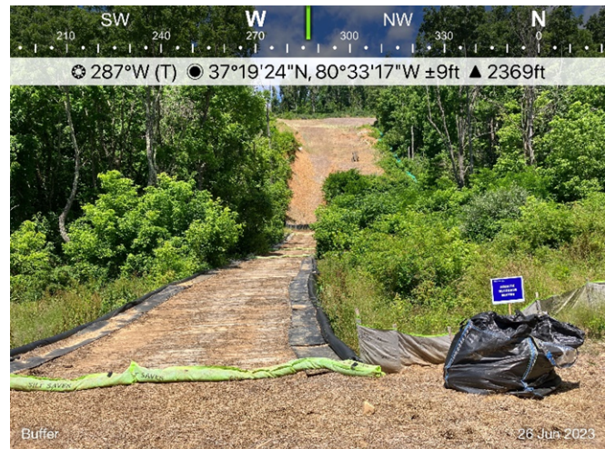
Figure 4: Designated crossings S-PA 07 & S-RR5, ECD's are in place.
