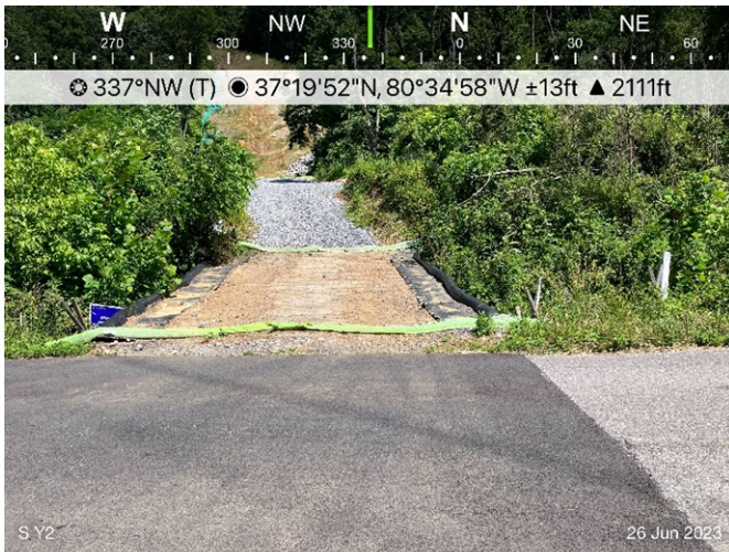
Figure 3: Designated Crossing S-Y2 ECD's are in place.
