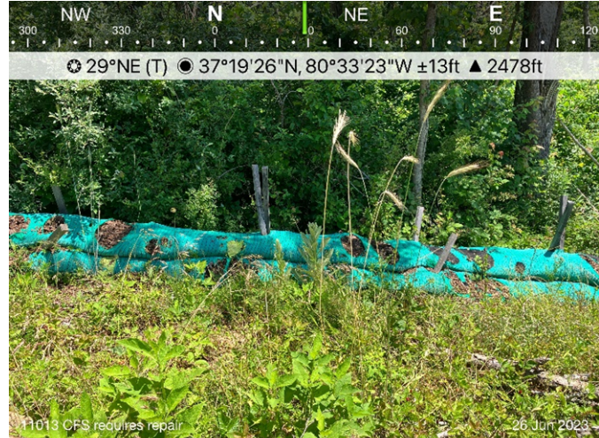
Figure 2: Sta 11013+00 CFS requires repair.
