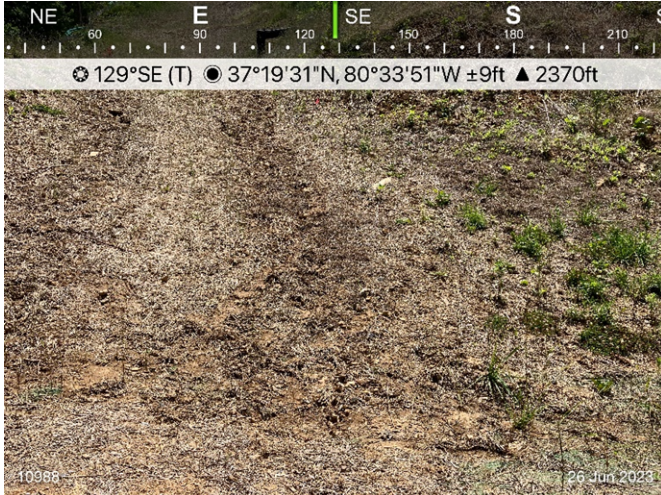
Figure 1: Sta 10988+00 rill erosion requires repair.
