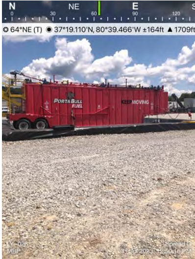
Figure 1: Laydown Yard 026 – Fueling station controls in place and functioning properly.
