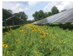
Gold Certified Cople Elementary School Solar Facility in Westmoreland, County (developed by SunTribe). Photo is after first growing season. Click to enlarge.
