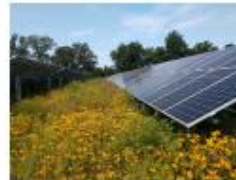
Gold Certified Cople Elementary School Solar Facility in Westmoreland, County (developed by SunTribe). (Photo is after second growing season. Click to enlarge. )
