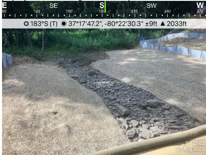
Figure 3: Stream S-EF62 – Controls in place and functioning properly. Stream crossing has been completed.
