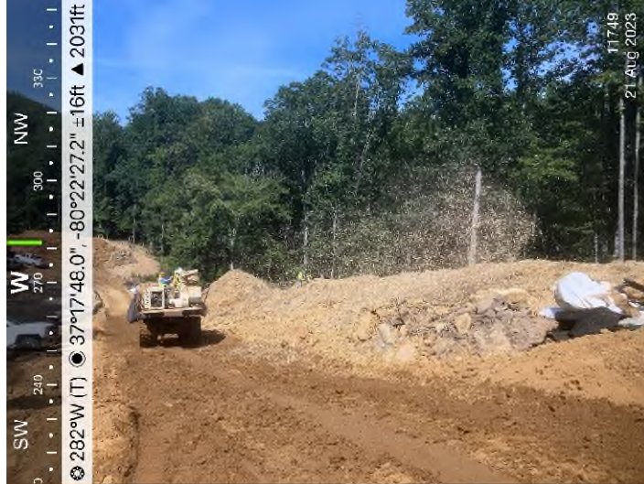
Figure 1: STA 11749+00 – Controls in place and functioning properly. Crews stabilizing stockpiles with straw mulch.
