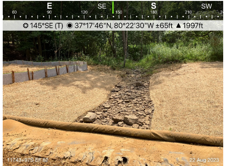
Figure 2: Designated crossing S-EF62, ECD's are in place.
