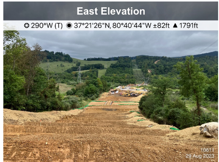
Figure 4: STA 10611, ECD's are in place.
