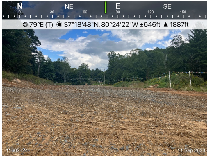
Figure 7: Sta 11602, ECD were in place.
