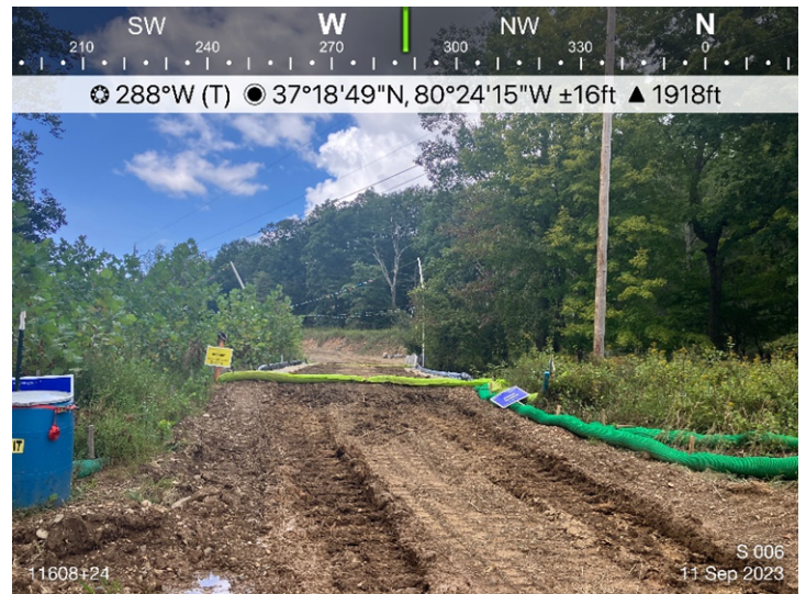
Figure 8: Designated crossing S-006, ECD's were in place.
