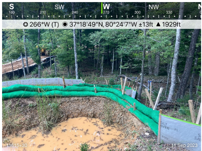
Figure 7: Sta 11615+30, ECD appears to be functioning above S-RR14.
