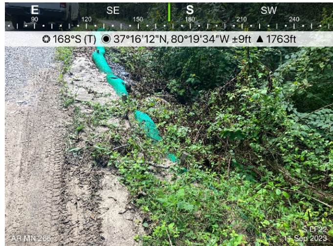
Figure 4: CFS requires cleaning/ maintenance along AR MN 266.
