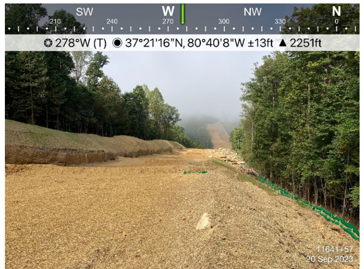
Figure 4: Sta 11641+57, ECD's are in place.
