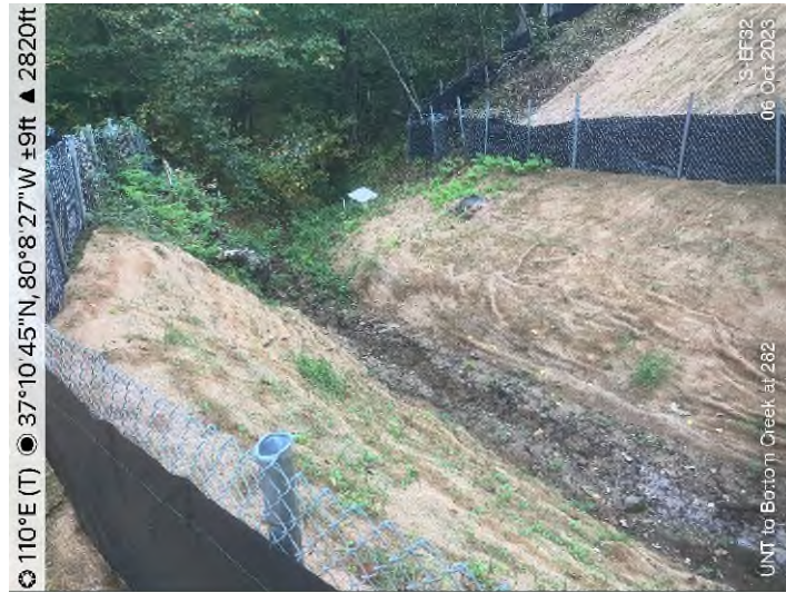
Figure 9: S-EF33 (UNT to Bottom Creek) – Conditions of UNT to Bottom Creek from the ROW crossing looking downstream within LOD.
