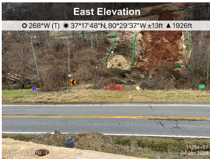
Figure 3: Sta 11254+57, ECD's are in place.
