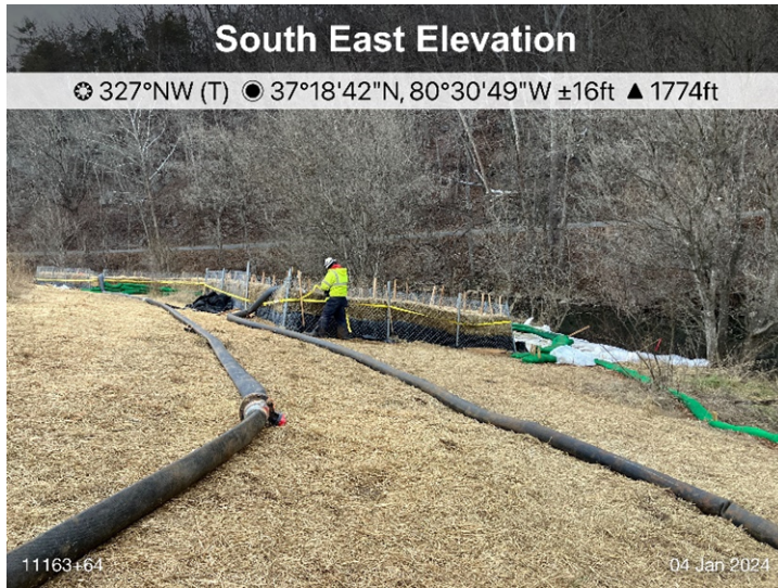
Figure 1: Sta11163+64, ECD's are in place.
