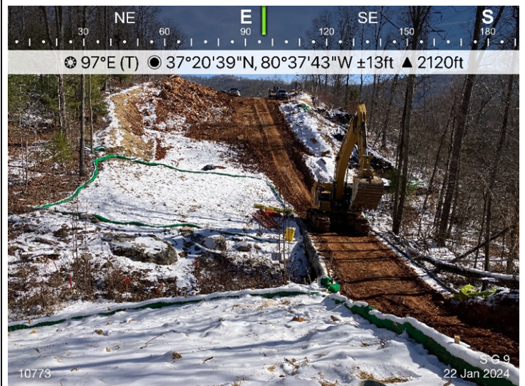
Figure 4: Designated crossing S-G9, ECD's are in place.
