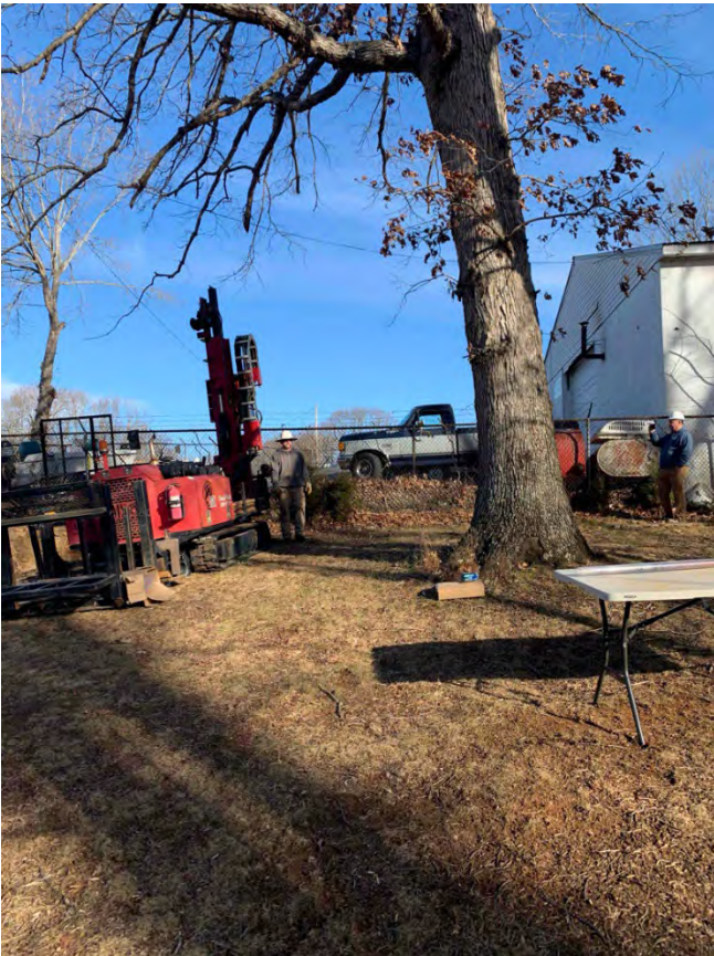
11. Boring B-2, south of the gasoline UST basin at 1640 Coopers Cove Road (12/22/2023)
