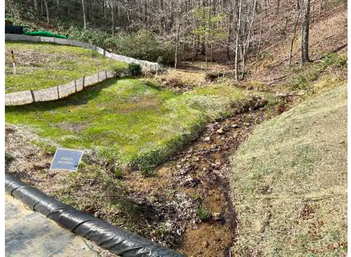
Figure 2: Stream S-MN21 – Controls in place and functioning properly.
