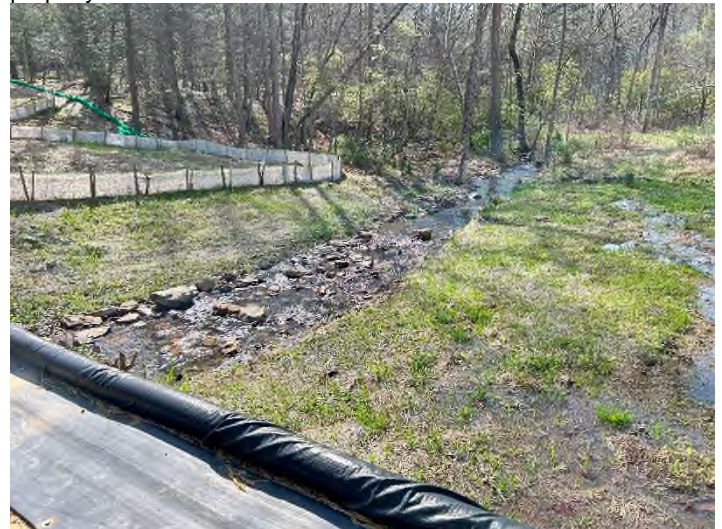
Figure 4: Stream S-EF62 – Controls in place and functioning properly.
