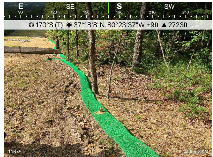
Figure 4: Sta 11675, approximately 30ft of erosion requires repair and re stabilized.
