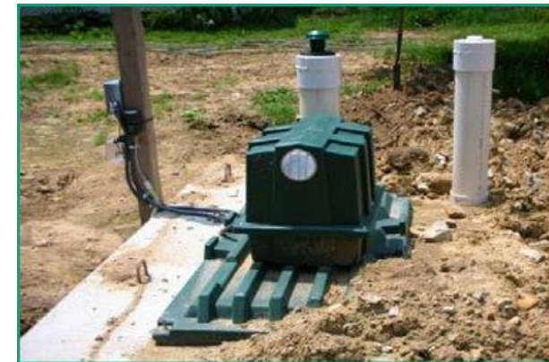
Alternative On-site Sewage Disposal System
