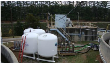
Figure 2. Pre-Post Filtration and GAC Units.
