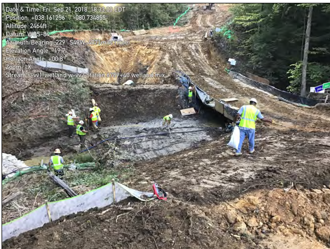
Photo illustrates the construction conditions of stream S-VV1 and wetland w-VV2. Note that the water has been completely diverted during construction.
