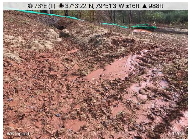
Figure 4: STA 14156+00 – Waterbar overtopped, repair needed.
