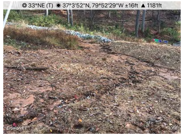
Figure 2: STA 14068+00 – Erosion depositing sediment into permanent waterbar rock end-treatment. Repair/stabilize erosion and remove sediment.
