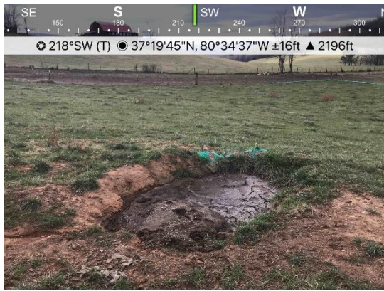
Figure 1: St 10948+50 sump requires sediment removal and CFS repair.
