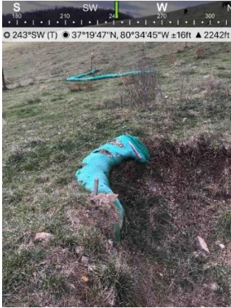
Figure 5: St 10942+22 sump requires CFS repair.
