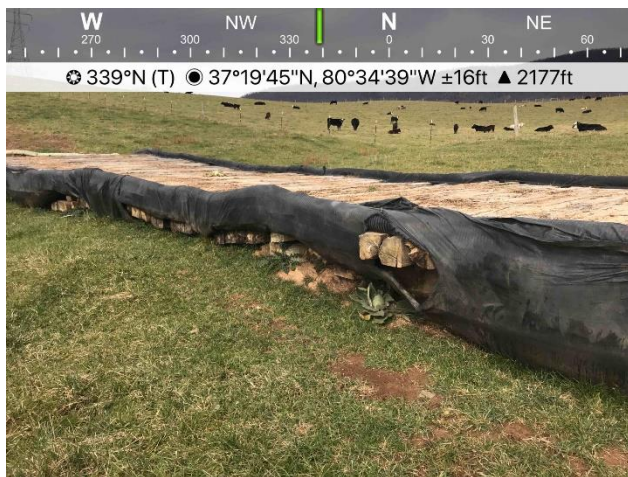
Figure 3: St 10947+00 bridge underlay fabric requires repair.
