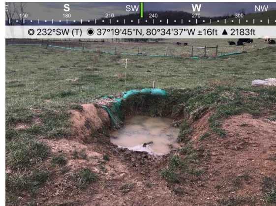
Figure 2: St 10947+50 sump requires CFS repair.
