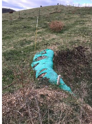
Figure 6: St 10941+00 sump requires CFS repair.
