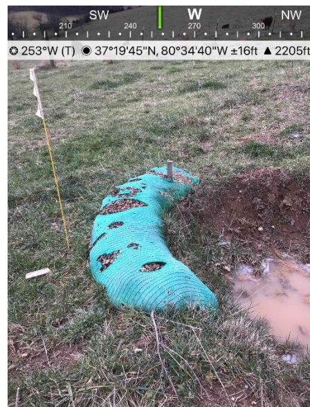
Figure 4: St 10946/10946+00 sump requires CFS repair.
