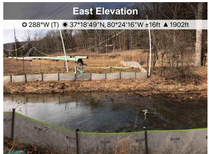
Figure 4: Designated crossing S-006, ECD's are in place and functioning.
