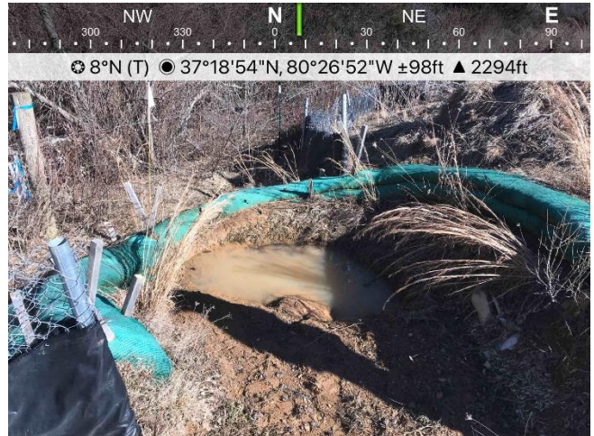
Figure 2: St11426 sump is at clean out level and requires maintenance.
