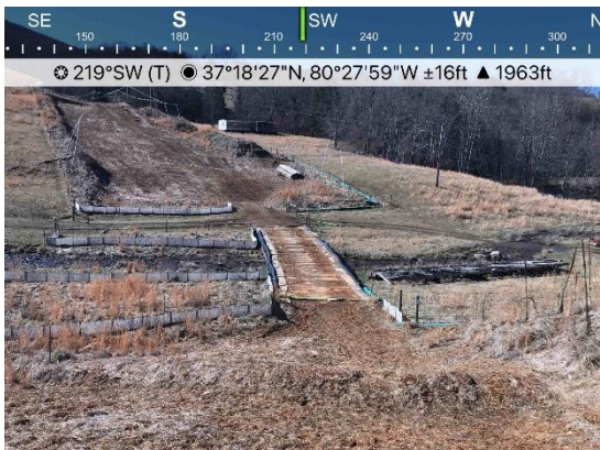
Figure 3: Designated stream S-KL43, ECD's are in place.
