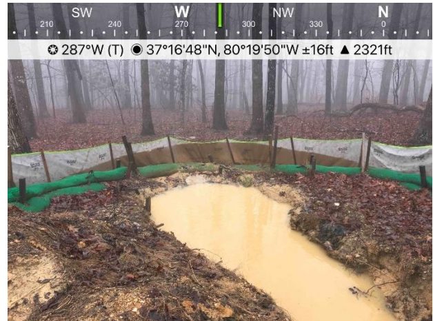
Figure 2: MVP inspectors have reported AR-MN266 sump maintenance.
