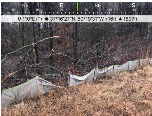
Figure 3: P1 is torn near St11960+00.
