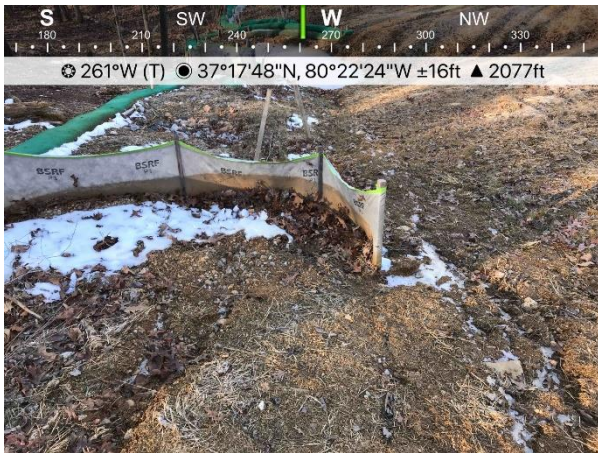
Figure 3: St11749+50 P1 requires sediment removal.
