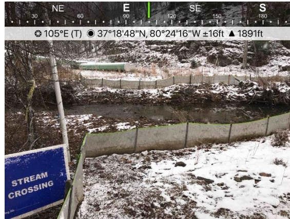
Figure 2: Designated crossing S-006 ECD's are in place.
