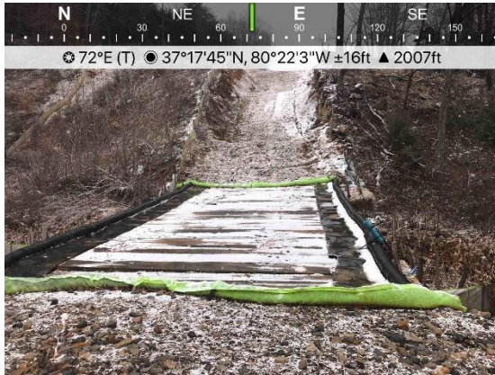
Figure 1: Designated crossing S-IJ52 ECD's are in place.
