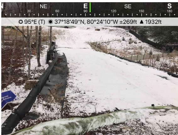
Figure 3: Designated crossing S-RR14 ECD's are in place.
