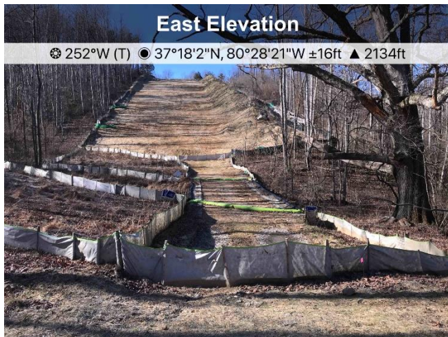
Fig. 3 At designated crossing S-NN12, ECD's are in place.
