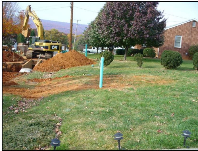
Figure 7.3. Photo showing home with failing septic system being connected to Western VA Water Authority sewer line (Photo: DEQ)
