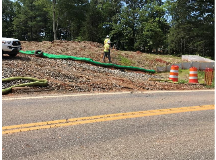
Stone construction entrance on north side of Brick Church Road clogged with mud
