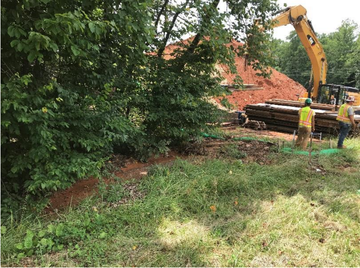
Sediment in roadside ditch.
