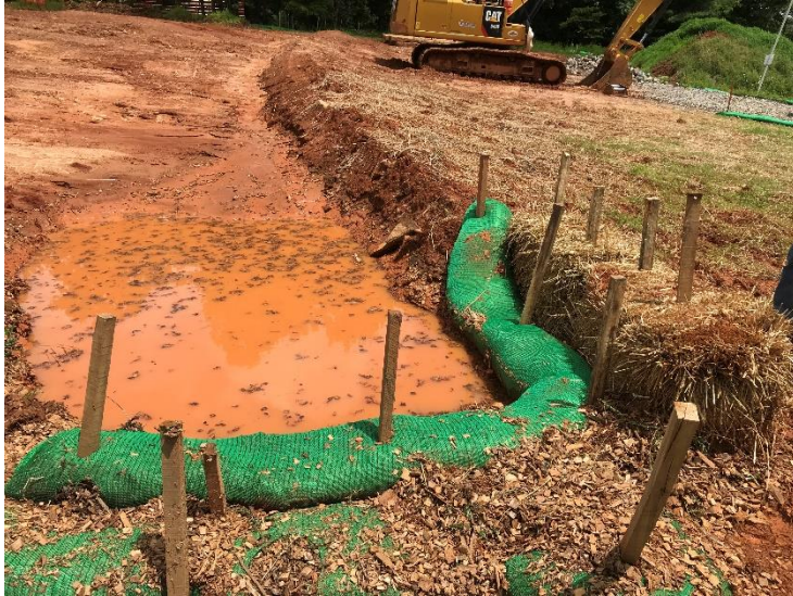
End of waterbar eroded, discharging downhill instead of off ROW. Repaired with straw bale.
