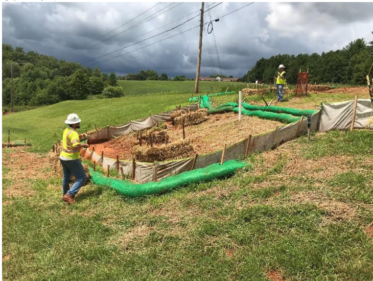
Silt fence loaded with sediment. Compost filter socks have sagged.
