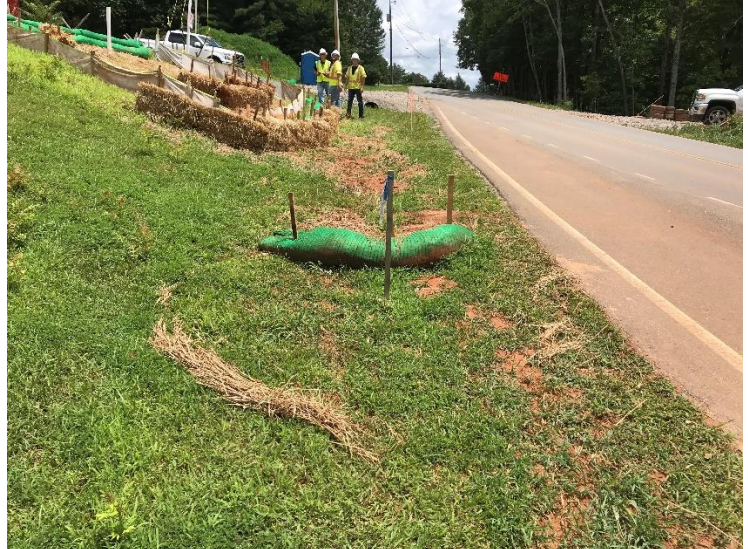
Filter sock check dam loaded with sediment. Sediment in roadside ditch.
