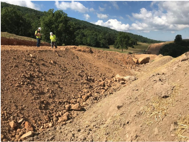
Side slope needs stabilization.
