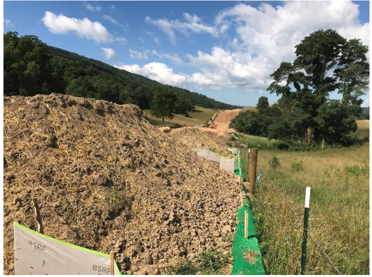
Stockpile needs stabilization, Filter sock needs cleaning out.
