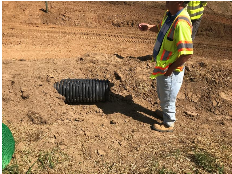
Pipe needs outlet protection
