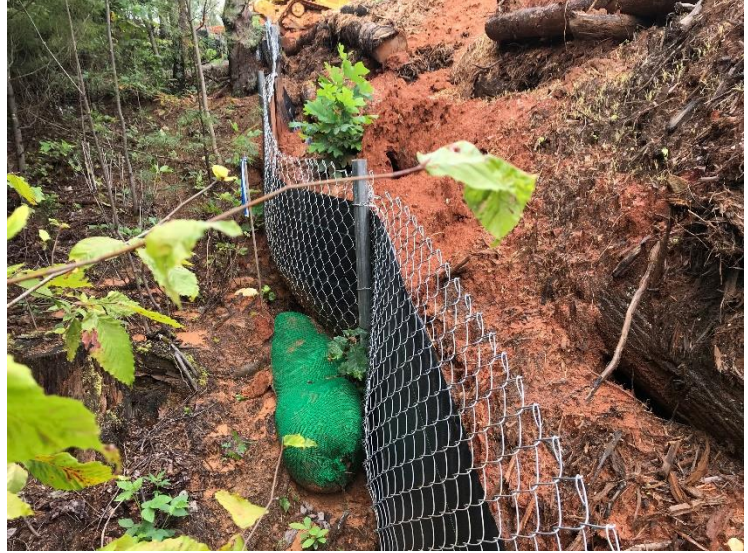
Silt fence undermined and discharging sediment off ROW.
