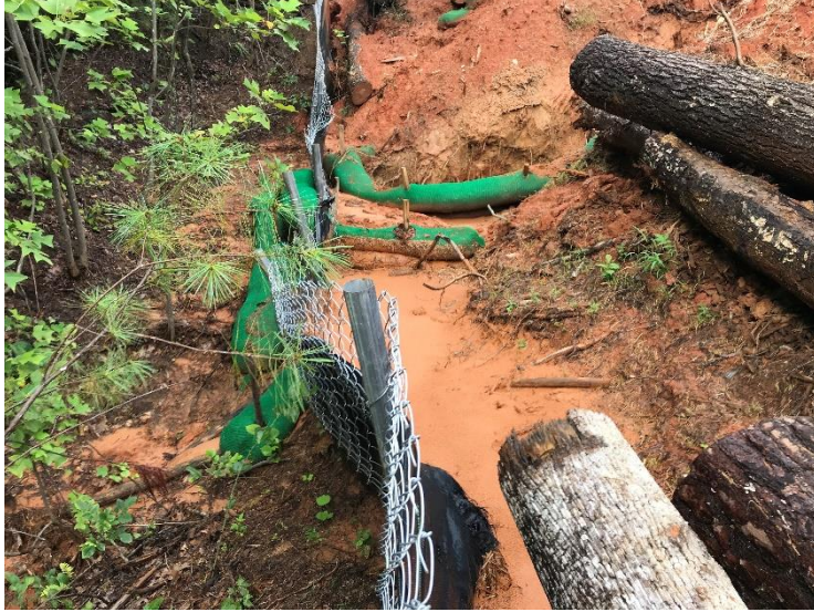
Waterbar end treatment full and discharging sediment off ROW
