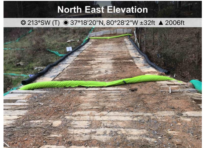
Fig. 2 Designated stream S-NN11, ECD's in place and functioning.
