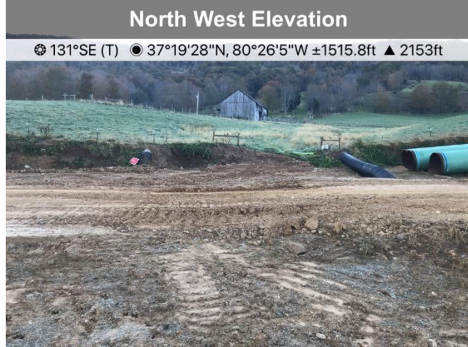
Fig. 1 At St# 11489 clean water diversion is inadequate.
