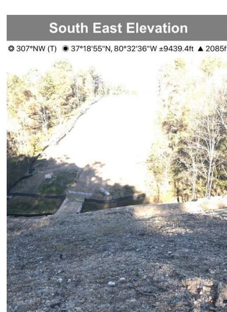
Fig. 2 St#11064+84-11073+00 is not adequately stabilized.
