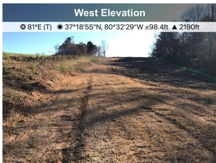
Fig. 3 St#11064+84-11073+00 is not adequately stabilized.
