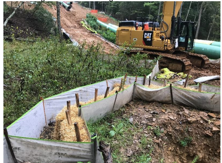
Fig. 4 Dewatering structure for designated stream S EF 65
