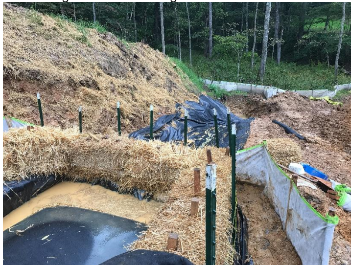
Fig. 3 Dewatering structure for designated stream S EF 65
