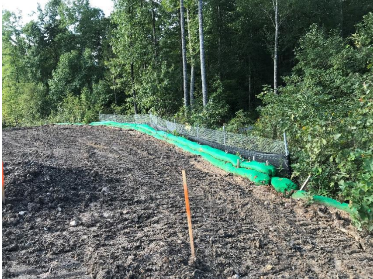
Fig. 1 MP 226.17 karsts feature protected
