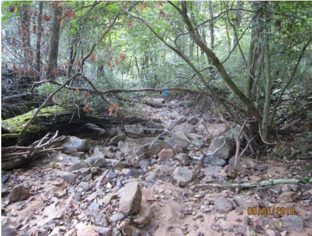
Photo 5: Sedimentation in channel 100' upstream of Rogers Road culverts; Depth = 8" Orientation: Upstream
