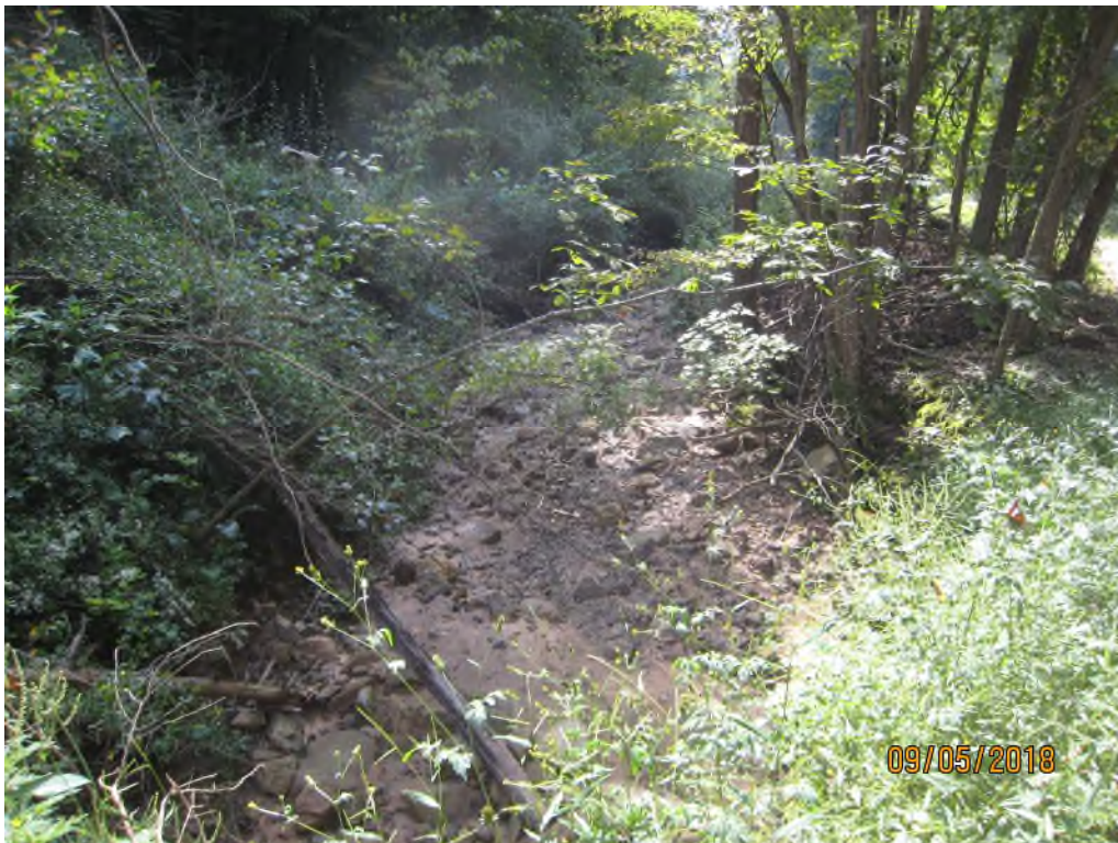
Photo 6: Sedimentation in channel downstream of Rogers Road culverts; no landowner permission Orientation: Downstream
