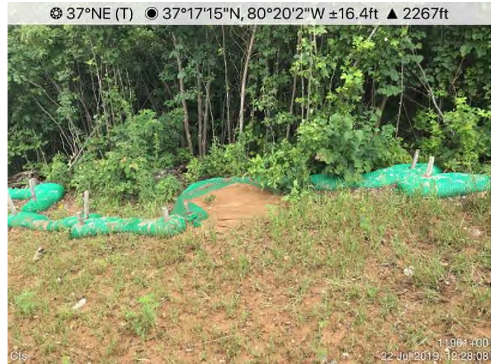
Fig. 6: STA 11901+00 – CFS maintenance needed.
