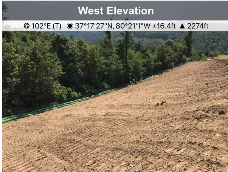
Fig. 1. Sediment was being removed at the time of the inspection at St 117833.
