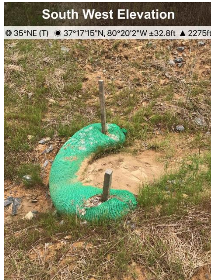
Fig. 1. Check dam on AR 266.03 requires maintenance
