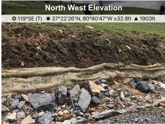
Fig. 1 Access Rd GI-234 matting has slipped off channel slope.
