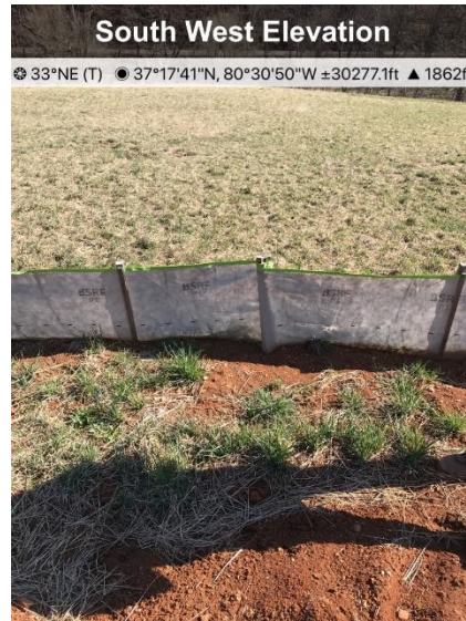
Fig. 2 St#11163+30 hole in P1 fence
