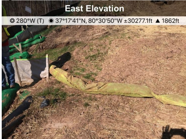
Fig. 1 St#11191+00 hole in bridge wattle
