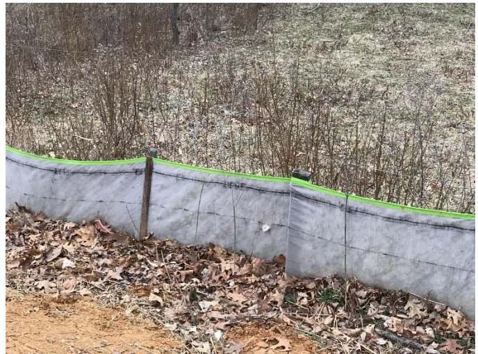
Fig. 4 St#11316+90 hole in P1 fence
