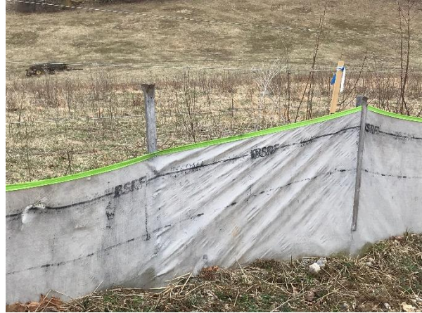
Fig. 2 St#11311+00 hole in P1 fence
