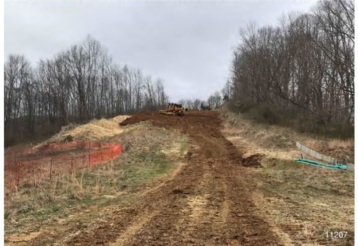
Figure 2: STA 11207+00 – Controls in place and functioning properly. BRG: 333°NW (T) LAT: 37.303751 LON: -80.506530 ±16ft ALT: 1957ft
