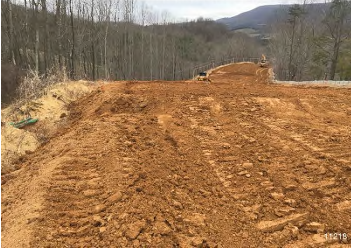
Figure 1: STA 11218+00 – Controls in place and functioning properly. BRG: 300°NW (T) LAT: 37.301381 LON: -80.503930 ±16ft ALT: 2080ft
