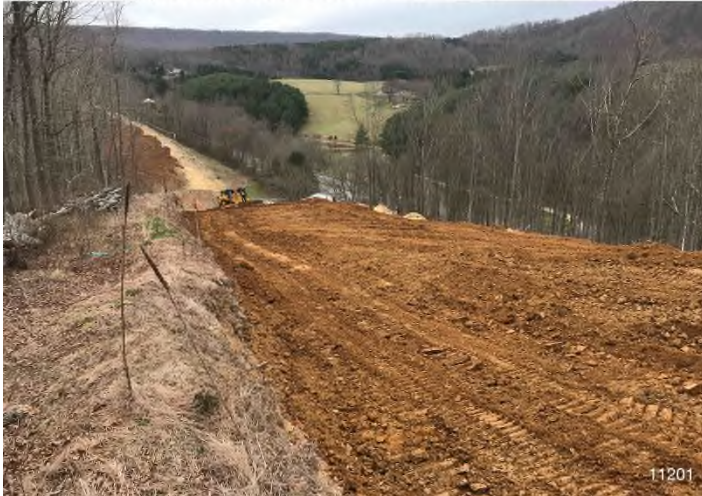
Figure 3: STA 11201+00 – Controls in place and functioning properly. BRG: 184°S (T) LAT: 37.305400 LON: -80.507007 ±32ft ALT: 2000ft
