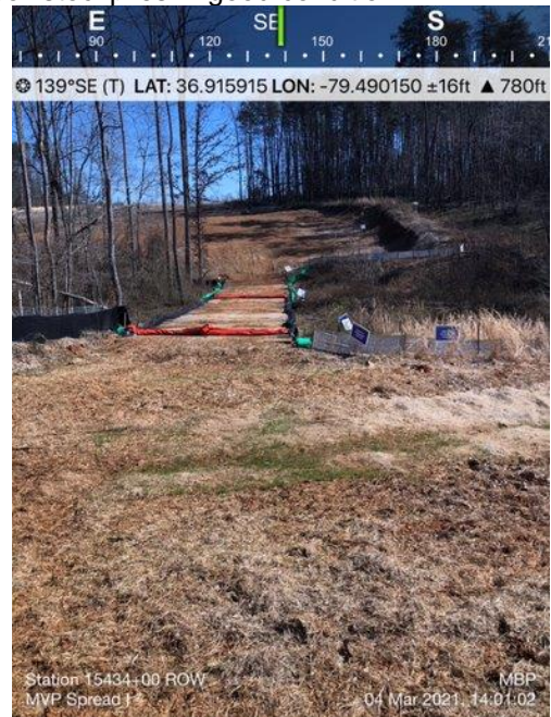
Photo 8. MBP Photo Mar. 4, 2021 showing E&S controls at stream crossing, stream buffer and stabilized topsoil stockpiles in good condition.
