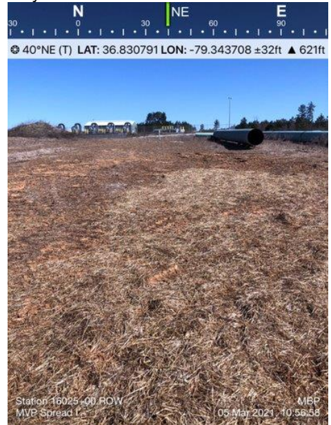
Photo 4. MBP Photo Mar. 5, 2021 at MP 302.1 showing poor vegetative cover with additional straw providing temporary stabilization.
