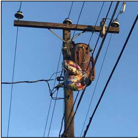
Figure 15: A photo depicting balloons in power lines, which can lead to power outages. Photo by Katie Register.
