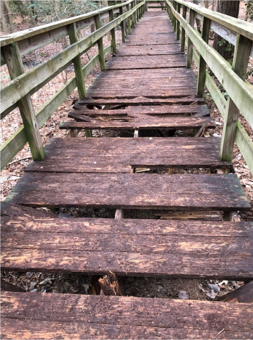
Photos of deteriorated walkway at Seaside “Park” aka the landfill in Northampton County.
