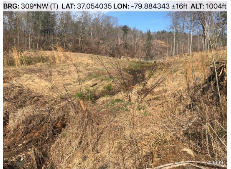
Photo 10. DEQ photo showing pond emergency spillway no longer discharging from the surface of the pond. .
