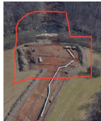
Milepost 269.4 DSC_0162 Inspection requested for apparent evidence of sediment runoff into stream and sparsely vegetated areas.
