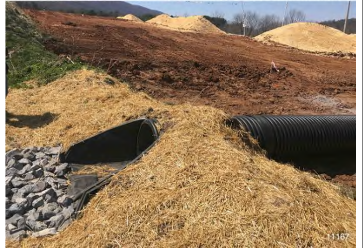
Figure 2: STA 11167+00 – PPL actively installing CWD and level spreader outlet. BRG: 240°SW (T) LAT: 37.310146 LON: -80.514244 ±32ft ALT: 1868ft
