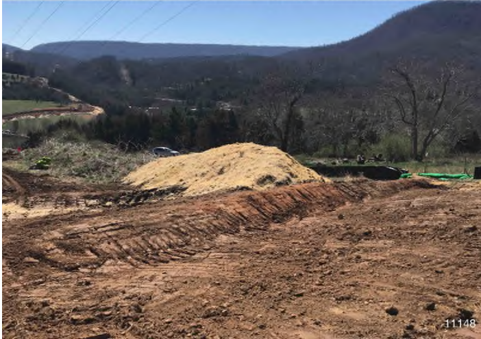
Figure 1: STA 11148+00 – Controls in place and functioning properly. BRG: 153°SE (T) LAT: 37.306572 LON: -80.509770 ±11398ft ALT: 1865ft
